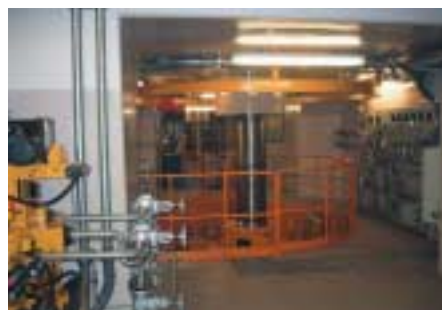
Interior view, powerhouse
