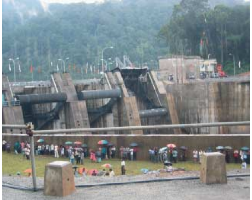
Dam with sectional gates
